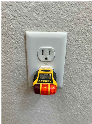
Electrical receptacles tested
