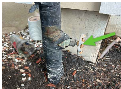
Main water shut off valve
