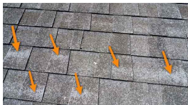
Shingle Granules Flaking Off
