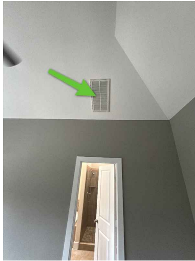
Air filter location-2nd floor
