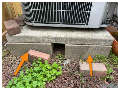
Improper Platform / Pad Support
