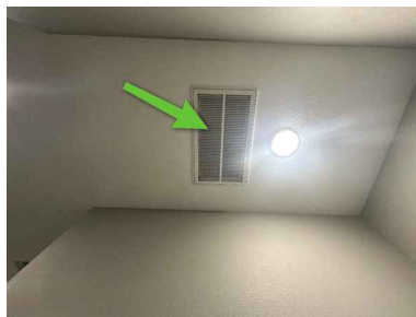
Air filter Location-1st floor
