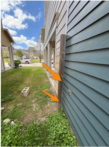
Wood Fence in Contact with Structure
