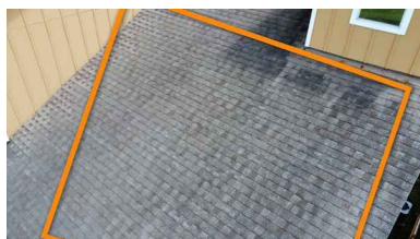
Shingle Granules Flaking Off
