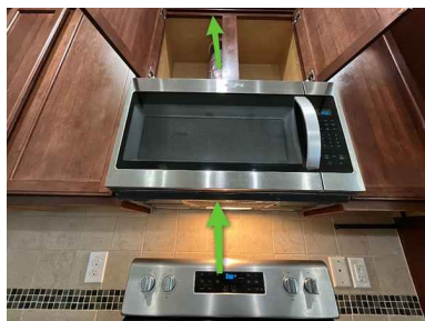
Range exhaust in operation
