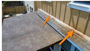
Roof Flashing Not Painted / Rusted
