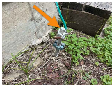
Ground Rod not Embedded
