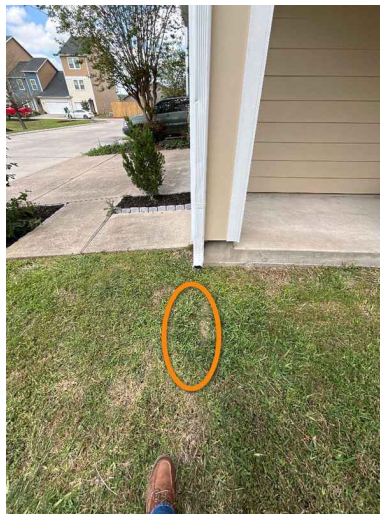
Splash Block / Extension Missing
