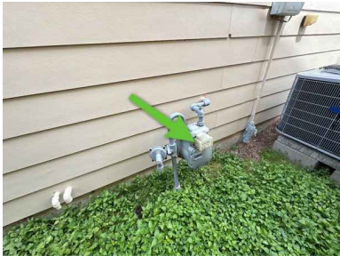
Gas meter location
