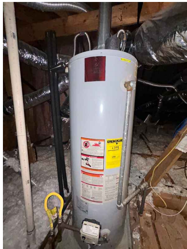
Water heater overview
