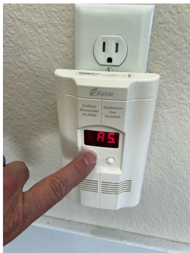
Carbon monoxide detector tested
