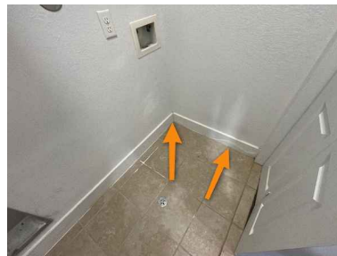
Flooring -Moisture Damaged
