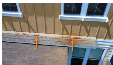
Shingle / Flashing Uplift
