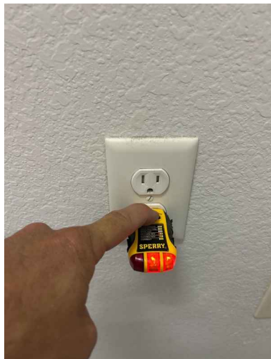
Missing GFCI Protection
