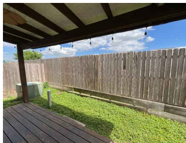
Damaged Fence Pickets
