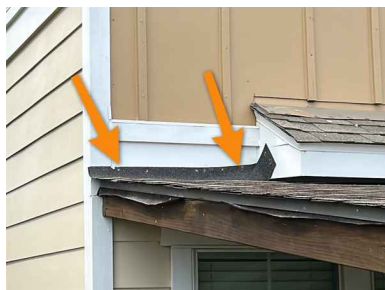
Missing Counter flashing
