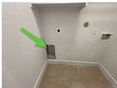
Dryer exhaust vent overview
