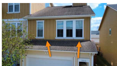
Shingle / Flashing Uplift
