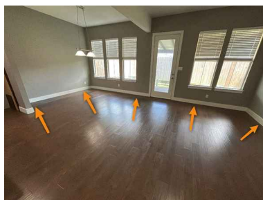
Flooring Not Sealed at Baseboard Interface
