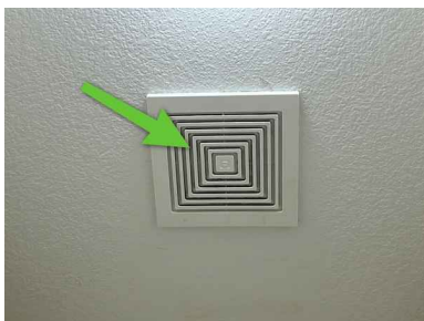
Mechanical exhaust vent in operation
