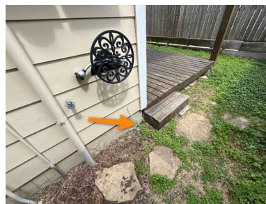
Ground Rod not Embedded
