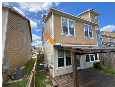
Missing Counter flashing
