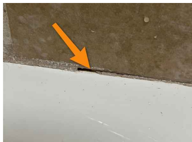
Missing/Damaged Grout or Caulking
