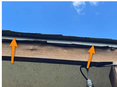
Roof Flashing Not Painted
