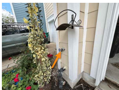
No Vacuum Breaker
