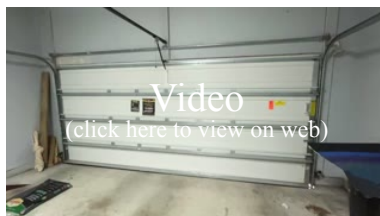
Garage door very hard to open and close
