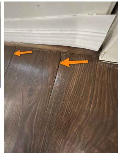
Flooring -Moisture Damaged
