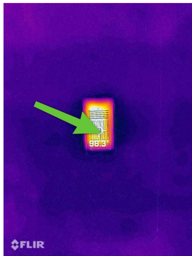
Furnace in operation-2nd floor
