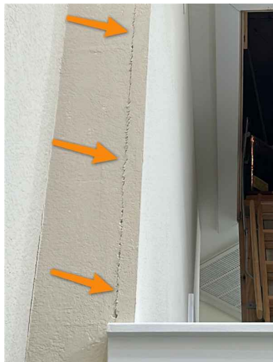
Peeling Cracked Texture
