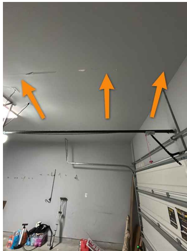
Peeling/Cracked Ceiling Texture
