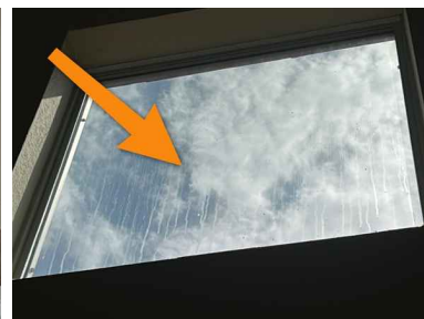
Failed Thermal Seal
