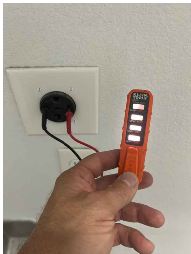
Dryer electrical receptacle tested
