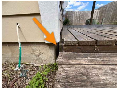
Deck separating from foundation
