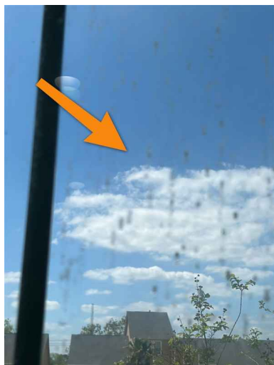
Failed Thermal Seal
