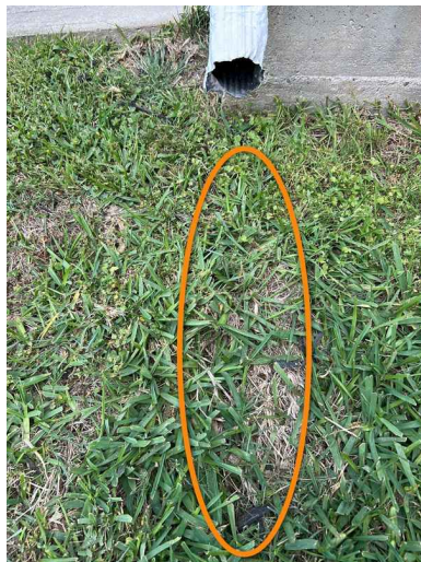
Splash Block / Extension Missing
