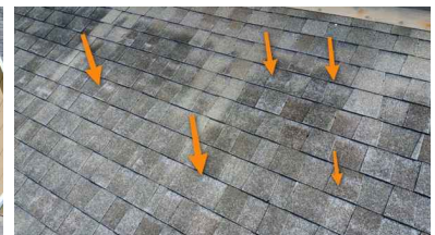
Shingle Granules Flaking Off
