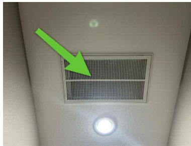
Return vents operated as intended
