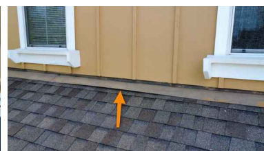
Shingle / Flashing Uplift
