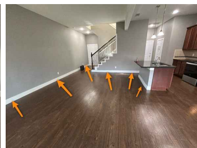
Flooring Not Sealed at Baseboard Interface
