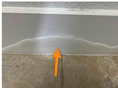
Flooring -Moisture Damaged
