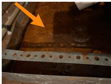
Moisture Observed in Overflow Pan
