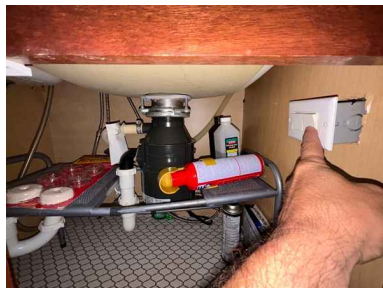
Food waste disposal in operation
