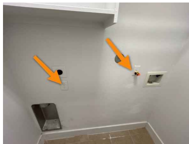
Missing GFCI Protection
