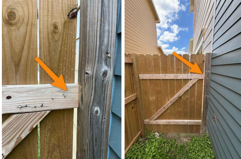
Fence Not Openable From Inside
