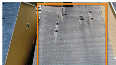
Shingle Granules Flaking Off
