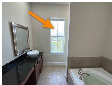
Failed Thermal Seal
