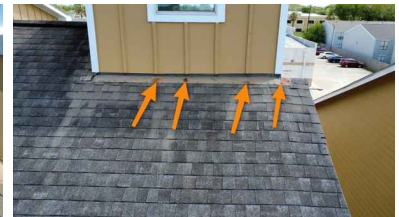
Roof Flashing Not Painted / Rusted
