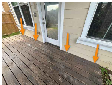
Counter flashing not installed
