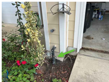
Main water shut off valve location
