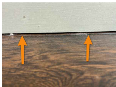
Flooring Not Sealed at Baseboard Interface
