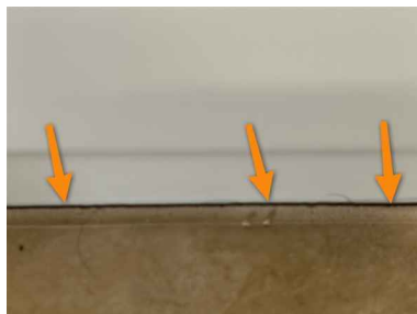
Missing/Damaged Grout or Caulking
