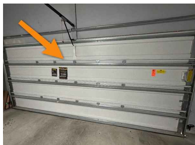
Garage door very hard to open and close
