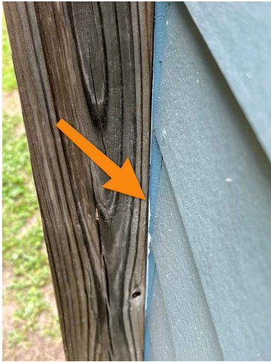
Wood Fence in Contact with Structure
