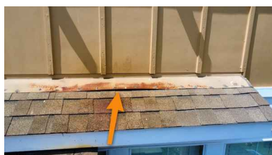
Shingle / Flashing Uplift
