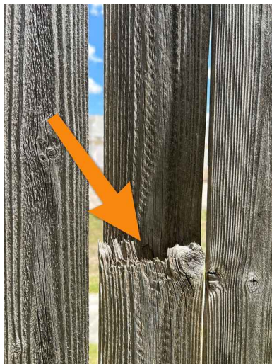
Damaged Fence Pickets
