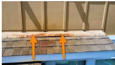
Roof Flashing Not Painted / Rusted
