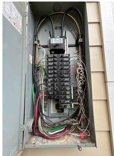
Main electrical panel overview
