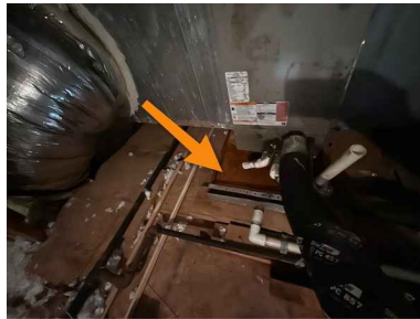
Rust in Overflow Pan
